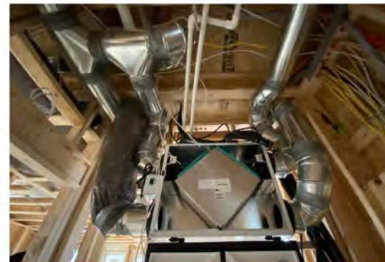
ERV in mechanical room
