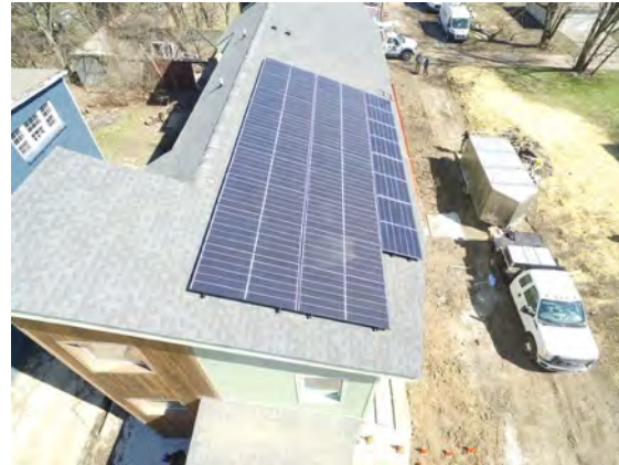
Jefferson Electric Solar
