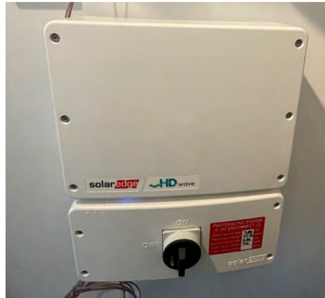
Solar Edge Inverter and power optimizer
