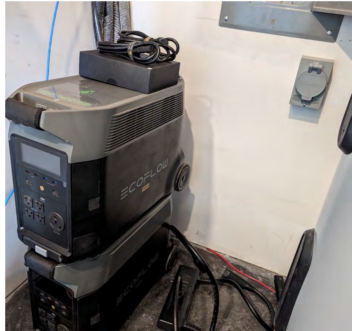
Battery backup system set up in the mechanical room
