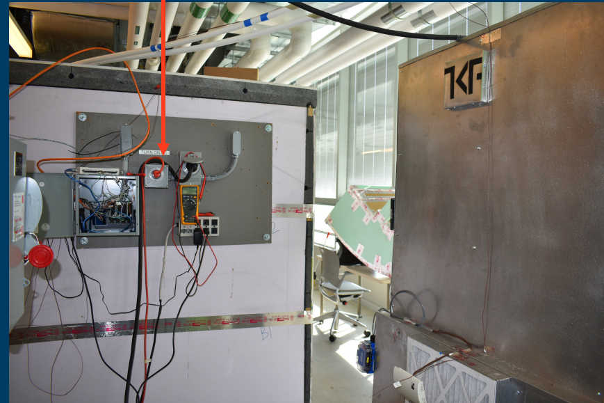
Power Monitoring and Test Controls
